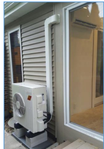
Figure 7: Ductless mini-split ASHP
